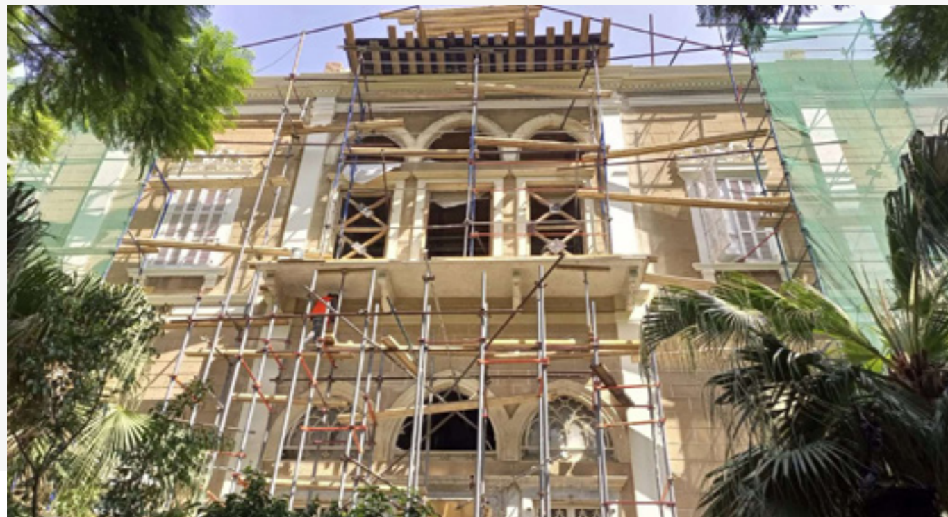
46 Photograph of Sursock Palace's South elevation, taken after finishing the lime plastering, painting the elevation, reproducing the extruded joints, grinding the marble slabs and cleaning the corbels.
